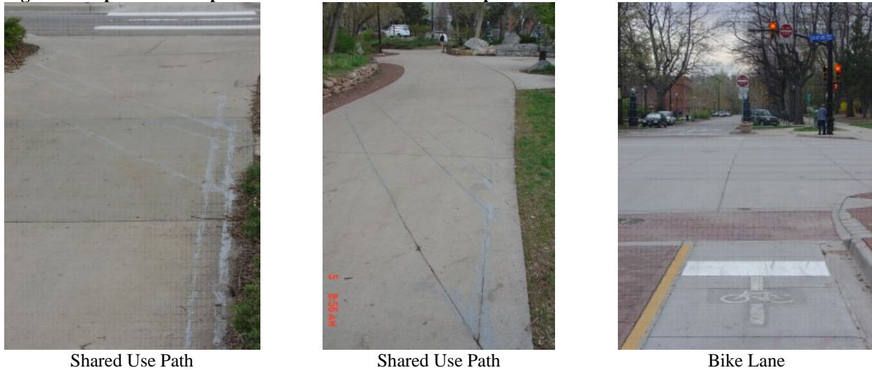
Figure 1. In-pavement loop detectors installed in shared use paths and bike lanes.
